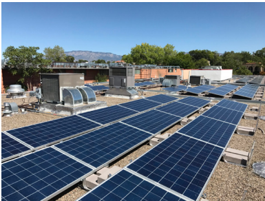
Solar Energy The warehouse's large roof area and site solar canopies will provide ample space for energy generation, potentially enough to generate all of the building's energy use requirements.
